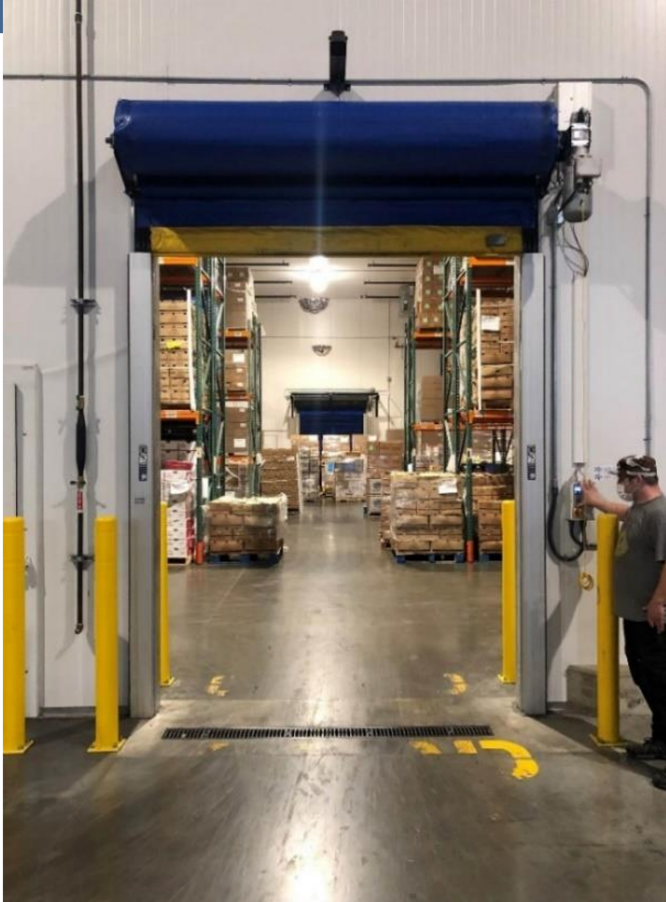
Cold storage facility (Food Lifeline)
